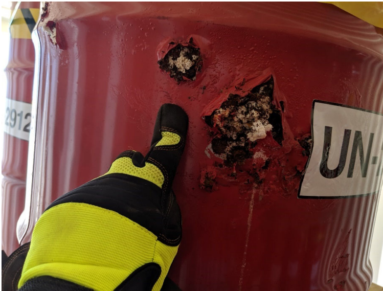
Figure 2 Corrosion of steel drum containing TENORM
