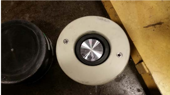
TU-1 Lead shield deformation
