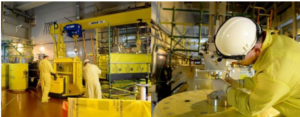
Figure 7: In order to minimise handling times GNS FAFNIR® and NEWA® were placed very close to each other in the Sizewell B Radwaste Building (left). Lifting the closure lid before connecting a MOSAIK® cask to the GNS FAFNIR® facility (right).
