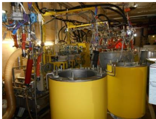
Figure 8: The GNS FAVORIT® plant ready to process ILW sludge in Bradwell's Circulator Hall 1.
