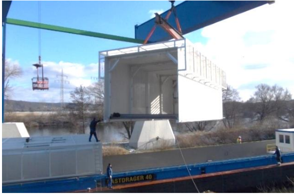
Fig. 6. River barge type LD40 during modification (lifting of component part of security enclosure).
