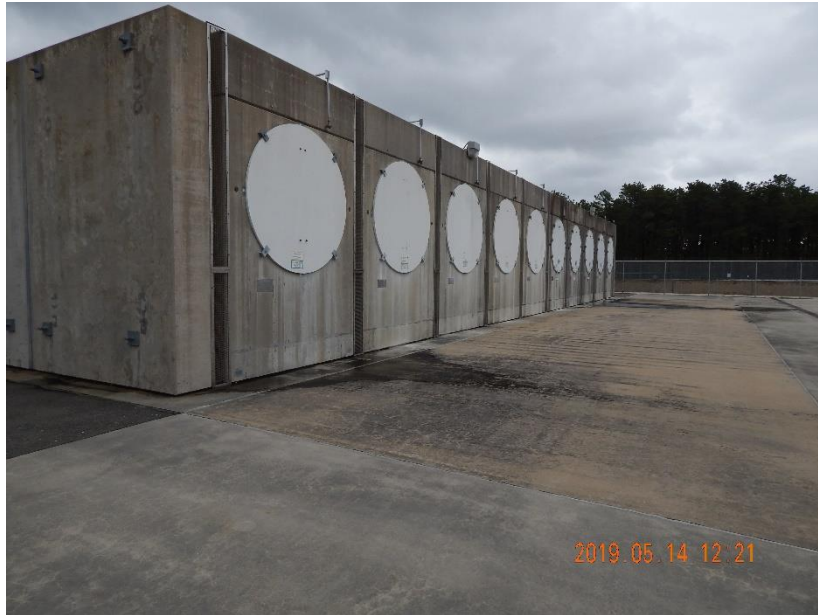
Figure 3 Oyster Creek Independent Spent Fuel Storage Installation (ISFSI)
