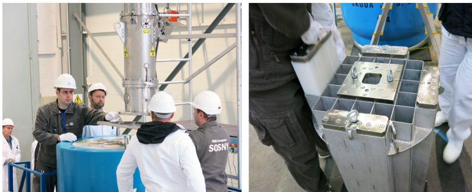
Figure 5 Equipment dry run to verify compatibility with SKODA VPVR/M cask
