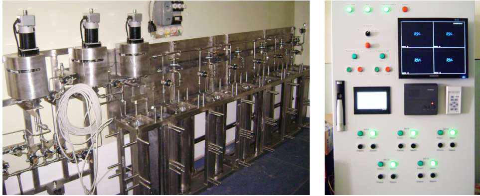
Figure 1 Partly-mounted equipment for liquid spent fuel discharge and temporary storage in the reactor hall
