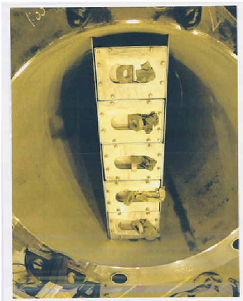
Figure 6, RWC with Waste Boxes (Courtesy of Exelon Corporation)
