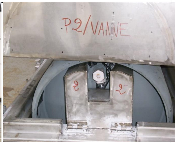
Figure 10: View of the valve
