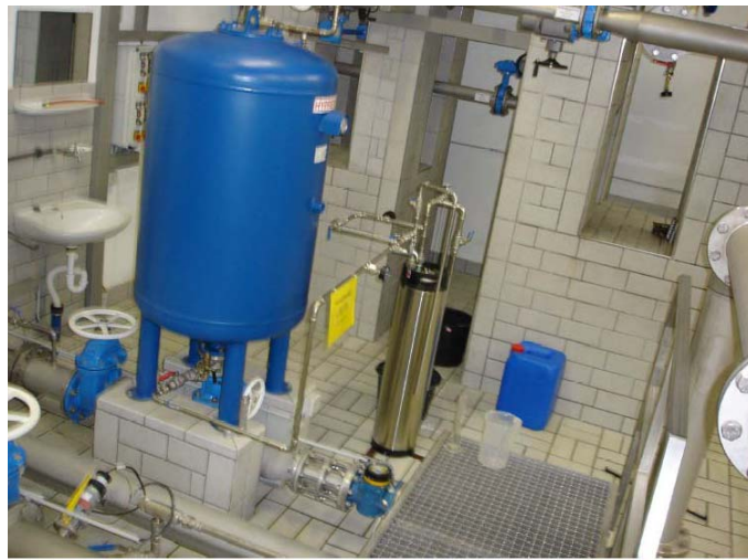
Figure 3. Filter system for the reduction of Uranium in potable water Uranium enriched Anion exchanger: up to 162 Bq/g U-238
