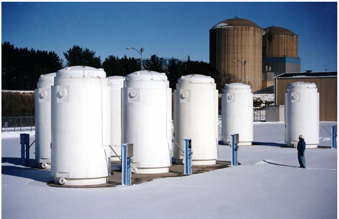
Figure 3 Representative Used Fuel Storage – NUHOMS® & TN Metal Casks
