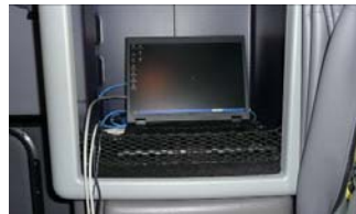
RJ45 line in cab
