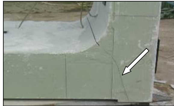
Figure 5. Crack at hollow section C3
