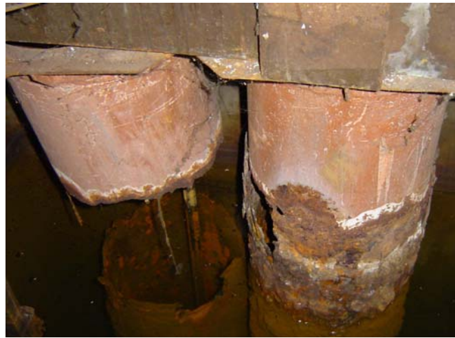
Figure 4. Corroded carbon steel components in Vinča spent fuel storage basin
