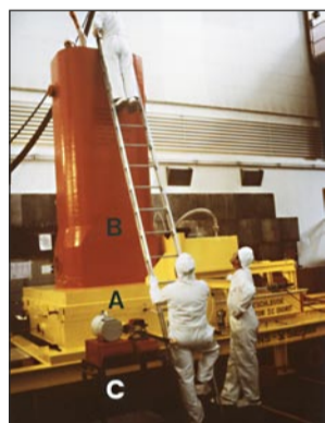
View of the Dry Loading of the Fuel by using: A) a mobile Transfer Cell B) a transfer Flask C) the CASTOR cask (bellow the transfer cell)
