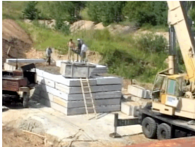
Fig.4. Stages to construct a target to conduct package impact tests, front part installation
