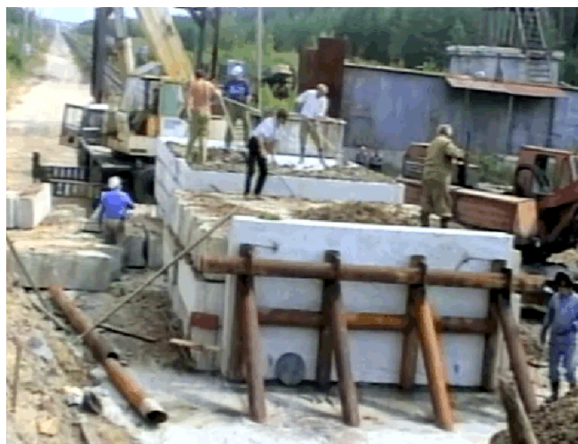
Fig.5. Stages to construct a target to conduct package impact tests, additional clamps of steel pipes
