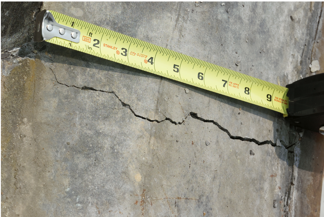
Fig. 4. Crack in top surface of shielding wall adjacent to impacted buttress.
