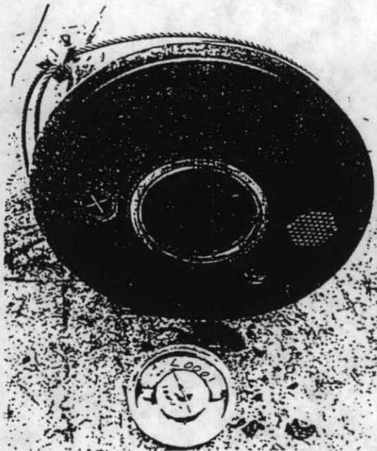
Fig 4. Grout lid detachment
