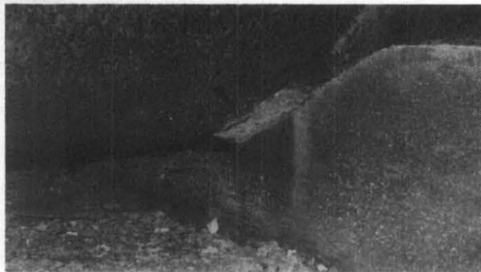
Fig. 6. Cylinders in storage at K-1066-K cylinder yard. Regions where accelerated corrosion attack might be anticipated are (a) lower head region, (b) areas in which dissimilar metals are in contact, (c) weld regions, and (d) areas where the cylinders rest on saddles. These regions are indicated with arrows.
