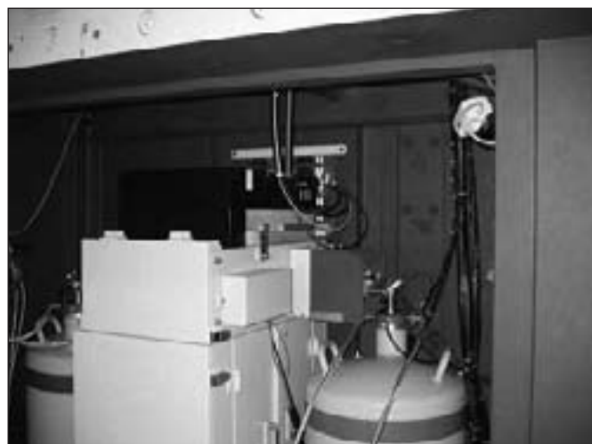
Figure 6. HKED-PNCC measurement station for input solution analysis at Rokkasho
