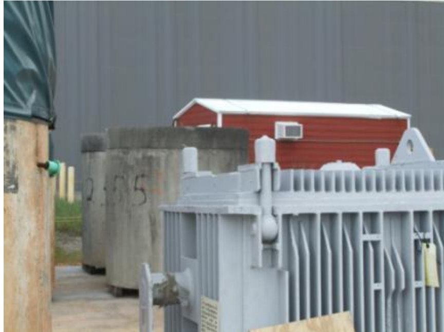
Figure 2 - Control Rod Cask (lower right)
