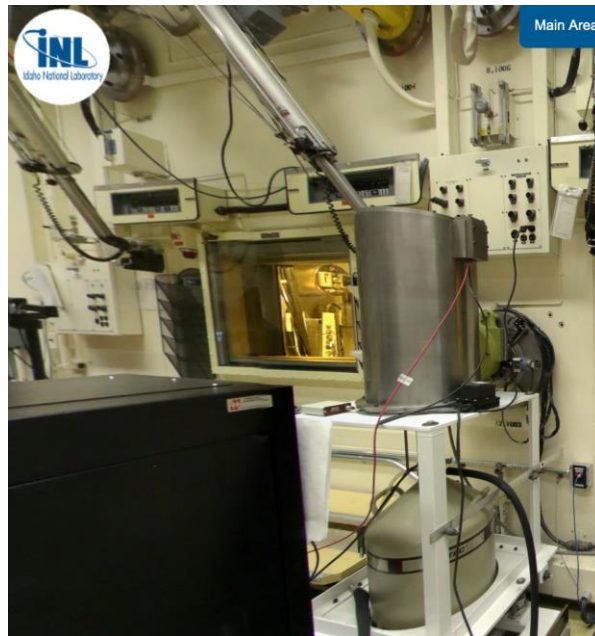
Figure 5: Germanium detector installed at Idaho National Laboratory’s Hot Fuel Examination Facility (HFEF) used to perform post-irradiation examination on irradiated fuel rods and specimens. The detector views items inside the hot cell through a collimator which reduces gamma flux and has a BGO guard detector to reduce effects from Compton scattering.
